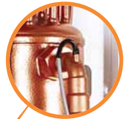
Flow & Return Sensors
